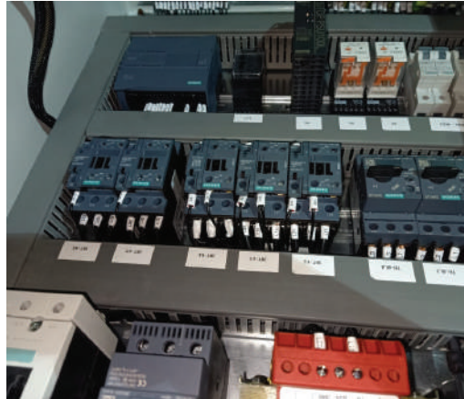
Automatic control systems
